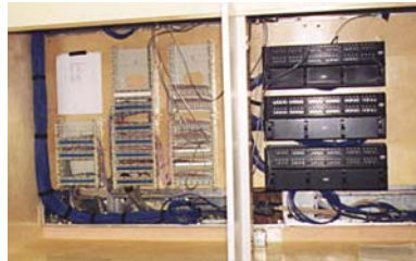
Wiring closet for voice/data patching
